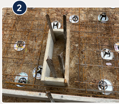
Hydrostatic valve void/cut out
