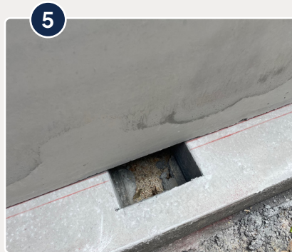
Placement of Plungie in relation to the hydrostatic valve void
